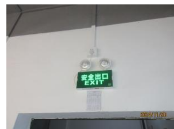
exit sign and emergency light.JPG
