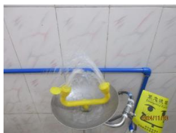
eye wash facility.JPG
